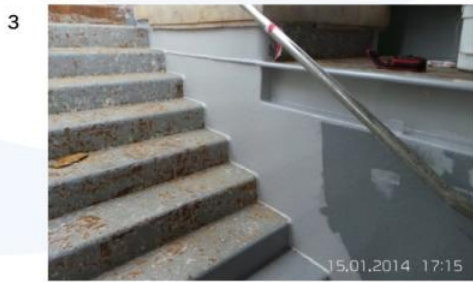
Photographs • Nos. 1-2 After Surface Preparation • No. 3 Topcoat Being Applied on Top of Primer
