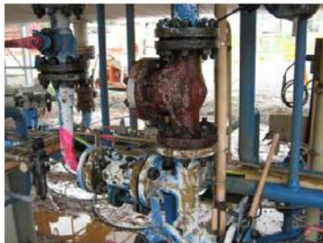
Before – Ammonia Bullet Pipelines
