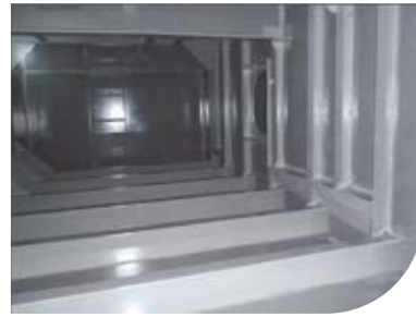
Potable Water Tank
