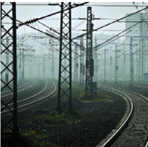
Stray Current Corrosion
