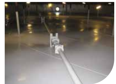
Crude Oil Tank
