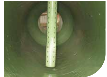
Hot-cote™ RD 900 Still Column Lining
